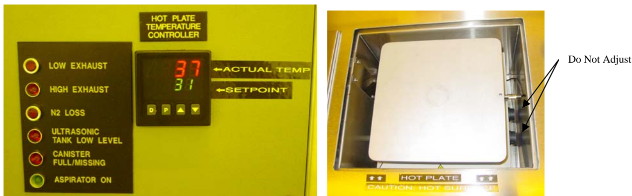
Figure 9. Recessed Explosion-Proof Hotplate, (Right), and temperature control and readout, (Left). See the knobs on the right side of the hotplate – Don't touch them!
