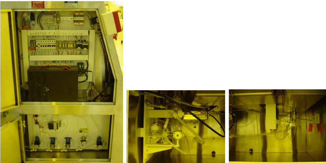
Figure 5. Hood Control (left) and plumbing facilities (right two photos). The large dark box in the middle of the left photo is the ultrasonic tank power supply.
