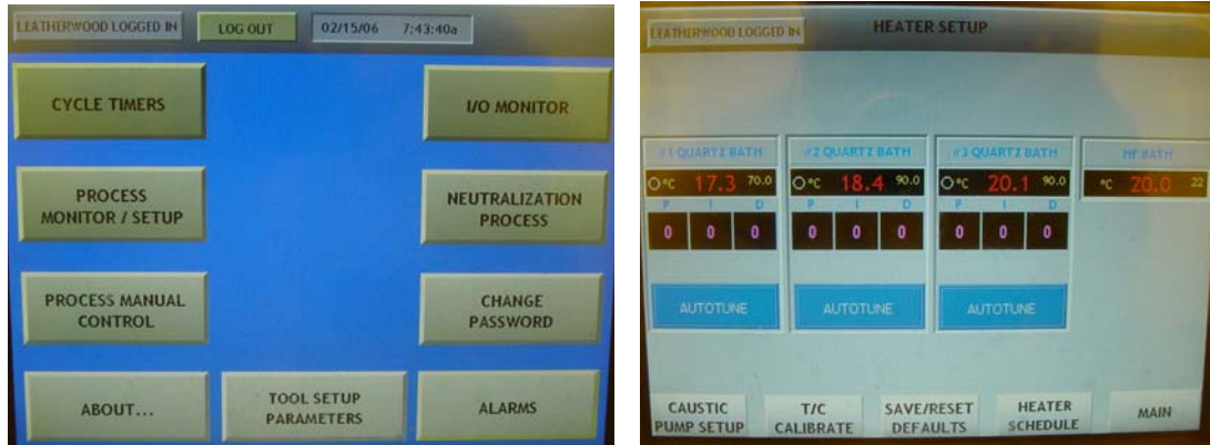
Figure A3. Software tree screens to find Caustic Pump Setup parameters.
