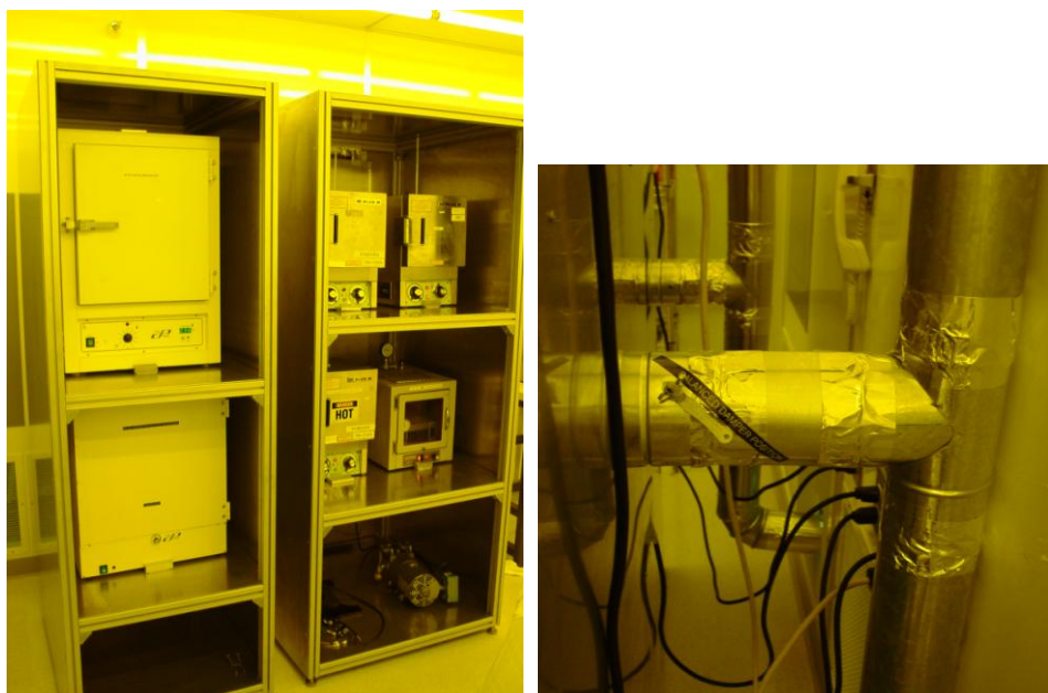
Figure 1. Blue-M oven enclosures, (left), and dampered exhaust connections, (right). Note the black diagonal label in the right photo depicting the proper angle for the damper handle.
