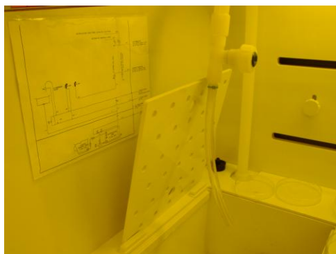
Figure 6. DI water sink accepts waste acids for neutralization.
