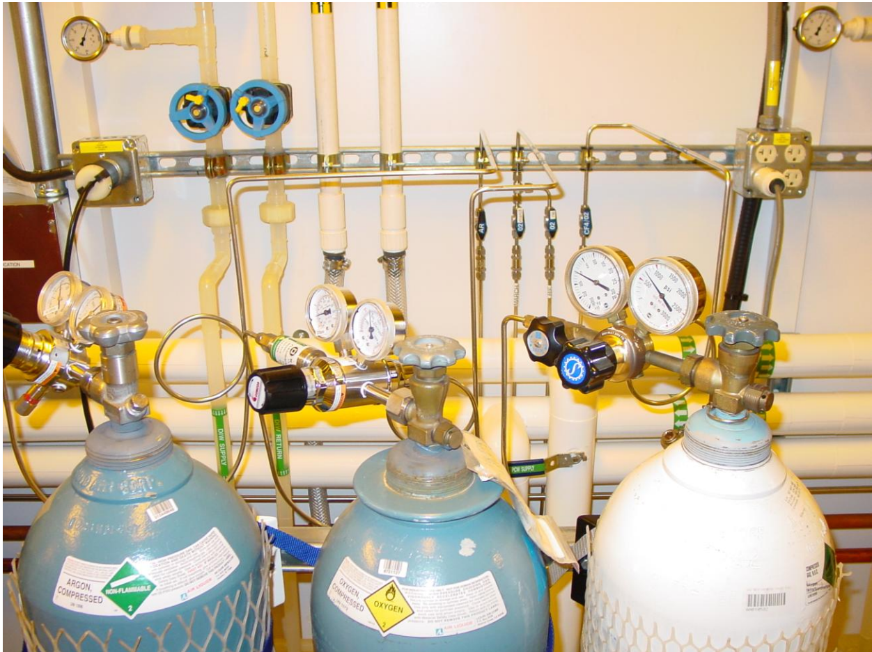
Gas and pump facilities are behind the chase wall and off limits to users.
